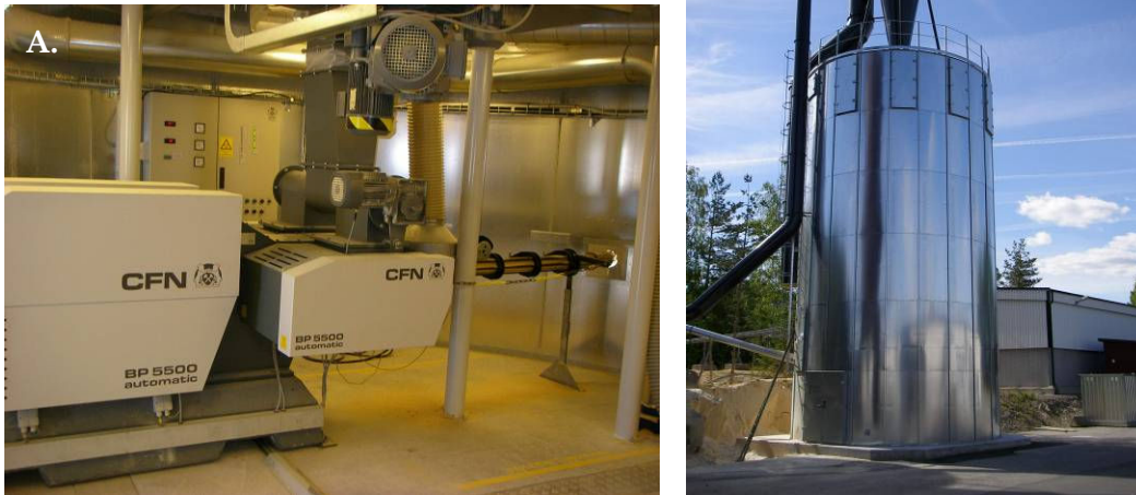
Figure 11. Briquetting and storage plant; a) C.F. Nielsen briquetter installed at base of silo; b) silo storage (Photo courtesy of Wayne Winkler).
