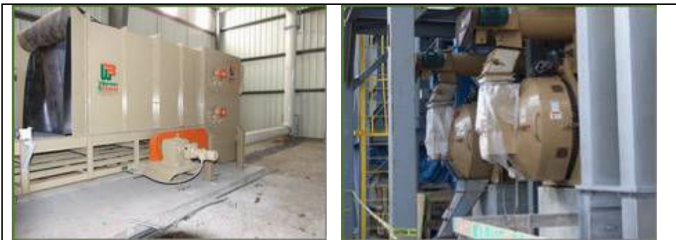
SMEC installed hay grind machine by Warren & Berg (left) and the Bliss Industries pellet mill ( www.goshowmeenenergy.com )
