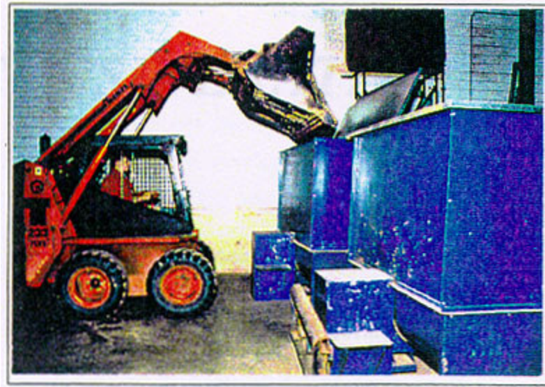
Bobcat loading woodchips into furnace hopper, (courtesy of Grove Wood Heat)
