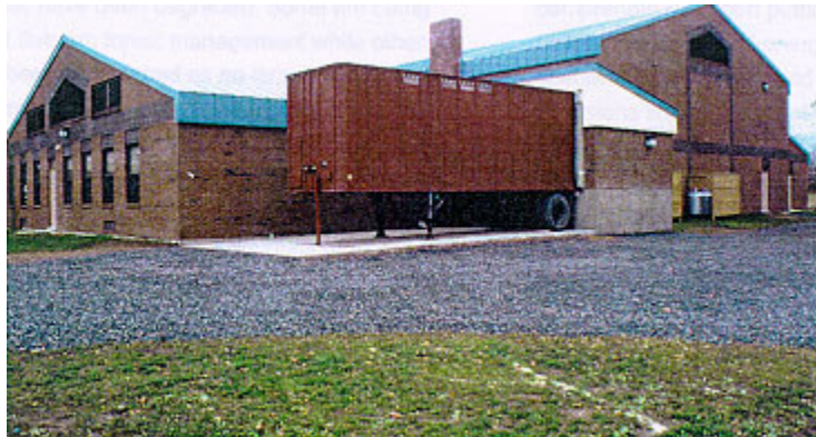
Woodchip heating installation at a Vermont school. Ten schools have been converted from oil or electricity to wood chip heating. (Courtesy of Chiptec Energy Systems)
